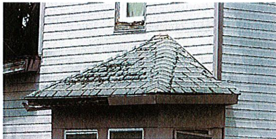
Roof in poor condition
