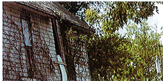
Hole in roof, wall open to interior.
