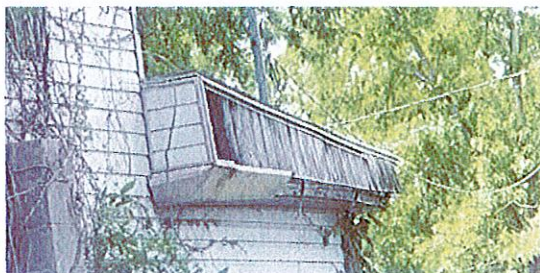
No paint or protection
